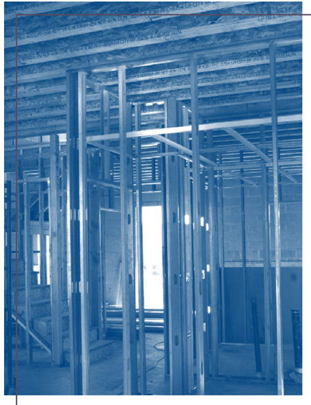
Steel framing is just one of many innovations currently being used in residential housing construction in the United States.
