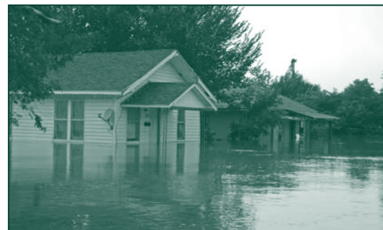
Flooded homes such as this one can be rehabbed safely for future use.
