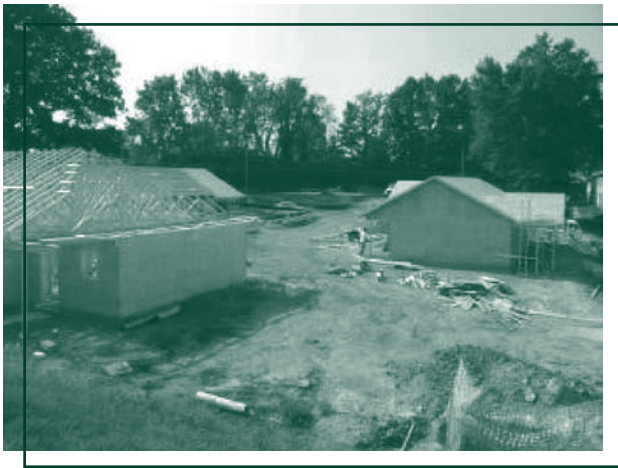
The Sapling Grove Apartments in Bristol, Virginia, will incorporate energy-efficient appliances, low-E glass windows, energy-conserving insulation, and high-efficiency heat pumps and water heaters.
