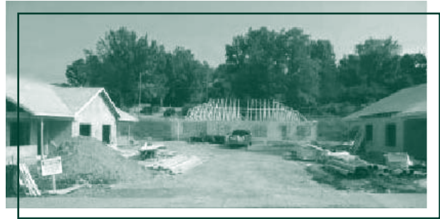
Residents will begin moving into the Sapling Grove Apartments in March 2008, with final occupancy planned for July 2008.
